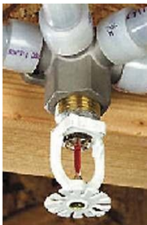
Fig 02. Sprinkler tipo quartzóid com defletor spray.
